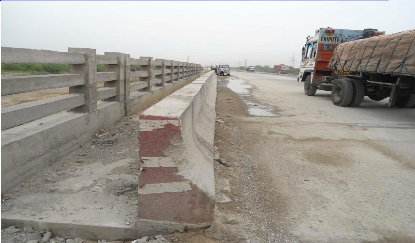
RCC Crash Barrier Hit by Vehicle
